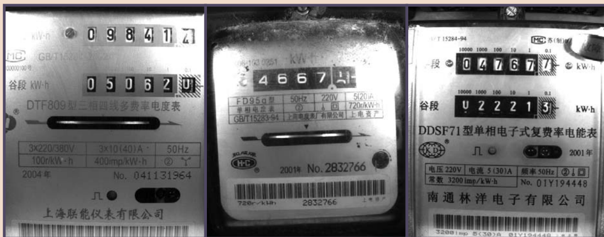
The differences in the meters brought challenges to the project. Note the meter in the center has 5 characters to read, while the others have 6. The center meter's right-side digit is between two values; the operator must manually record this reading.
